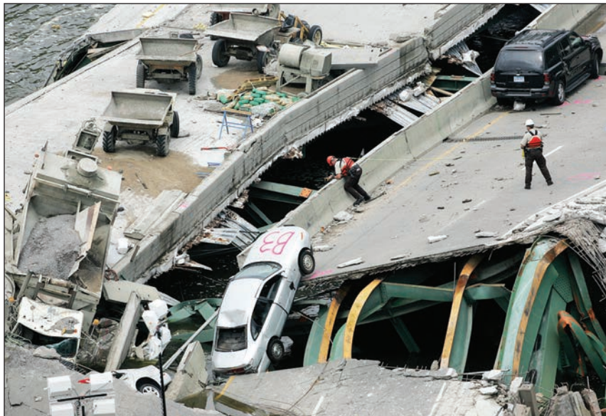
Rescue crews search under a collapsed bridge on Interstate 35 in Minneapolis, August 5, 2007.
