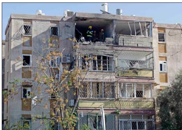
Three people were killed when a rocket hit this building in southern Israel.
